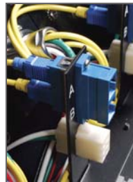
Internal SC and electrical breakout
